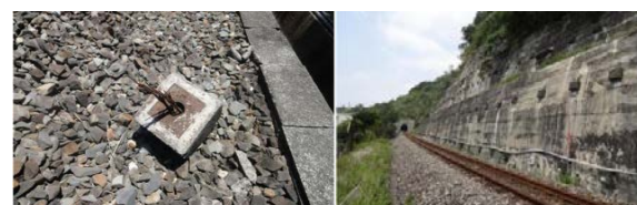
(c) 錨頭掉落
