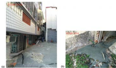
FIGURE 9 (a) the most settled house in Tainan due to 0206 earthquake-induced soil liquefaction. (b) The excessive sand boiling observed around the house.
